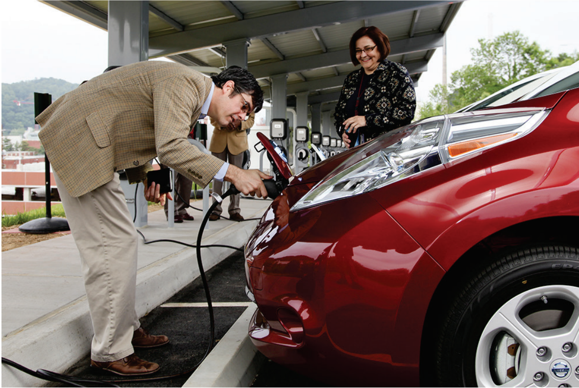
Fig. 5.8. ORNL’s solar-assisted electric vehicle charging station.
