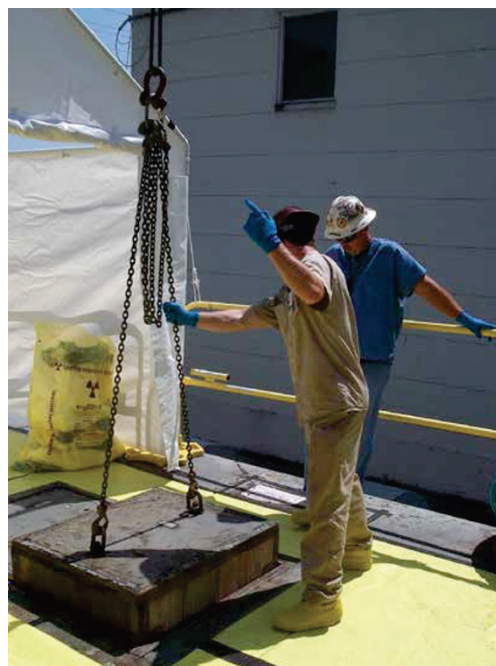
Fig. 5.44. HEPA shield plug being removed from a filter pit.
